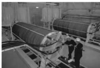
(b) Two 200Nm 3 H 2 /h alkaline electrolyzers each functioning at atmospheric pressure, from Norsk Hydro (photo taken from [KRU 02])
